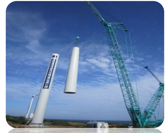
Phu Quy Windfarm Project
